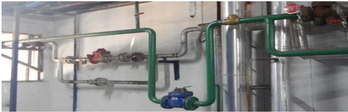
Figure 2. Installed Piping and Fittings before the Modification
